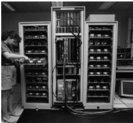
Figure 3: The physical packaging of the RAID-II File Server. Two outer racks contain 144 disks and their power supplies. The center rack contains three chassis: the top chassis holds VME disk controller boards; the center chassis contains XBUS controller boards and HIPPI interface boards, and the bottom VME chassis contains the Sun4/280 workstation.
